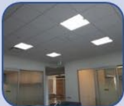
Troffers, Office, Classrooms
